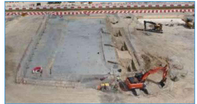
Transformer Yard and Relay Building
